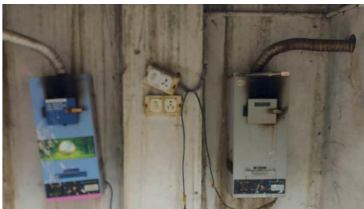
Sanitary Napkin Incinerators at Girls Hostels
